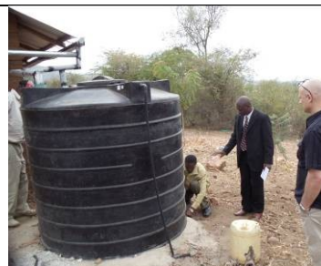
New water tank; note the piping from the roof
